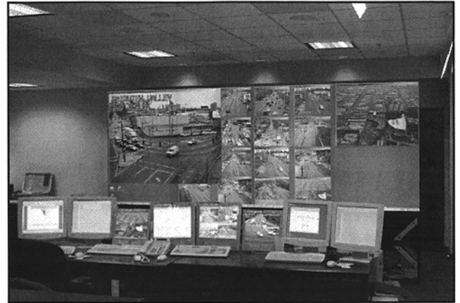
Duwamish ITS Control room.
